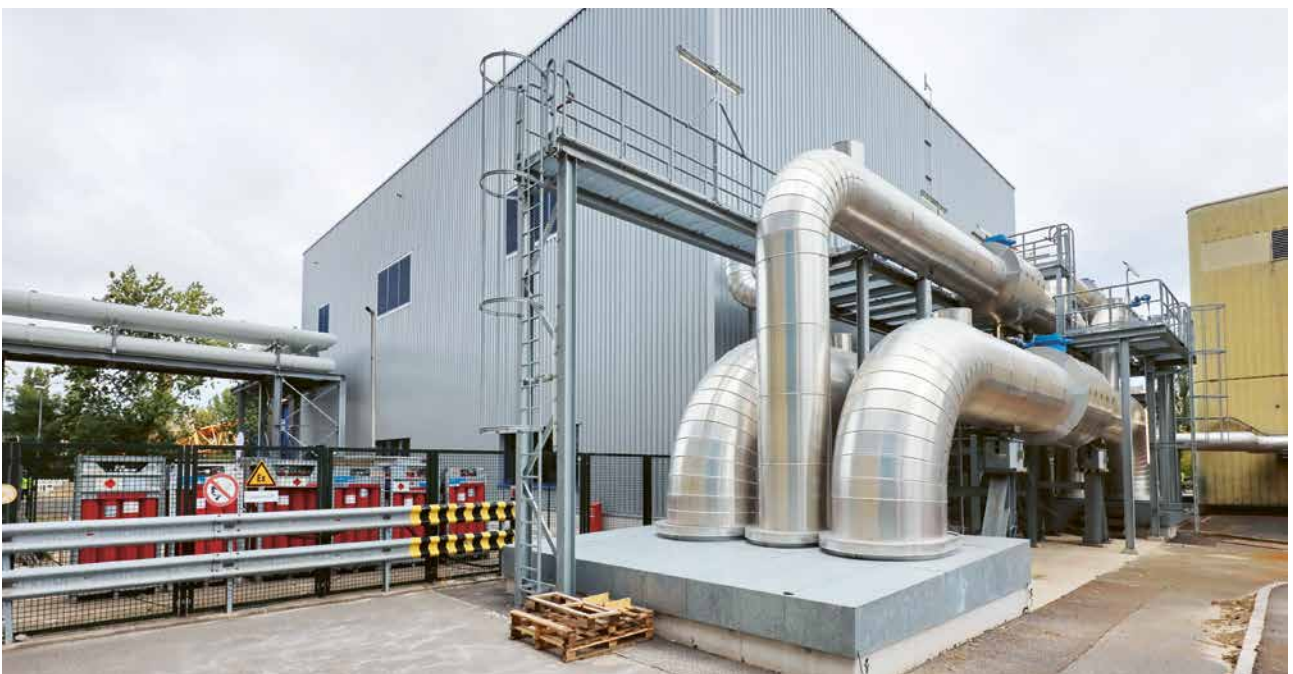
▼ Exterior view of the Power-to-District-Heating site.
