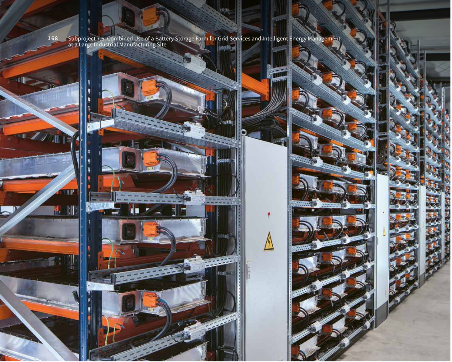
▲ Interior view of the BMW battery storage farm in Leipzig.
