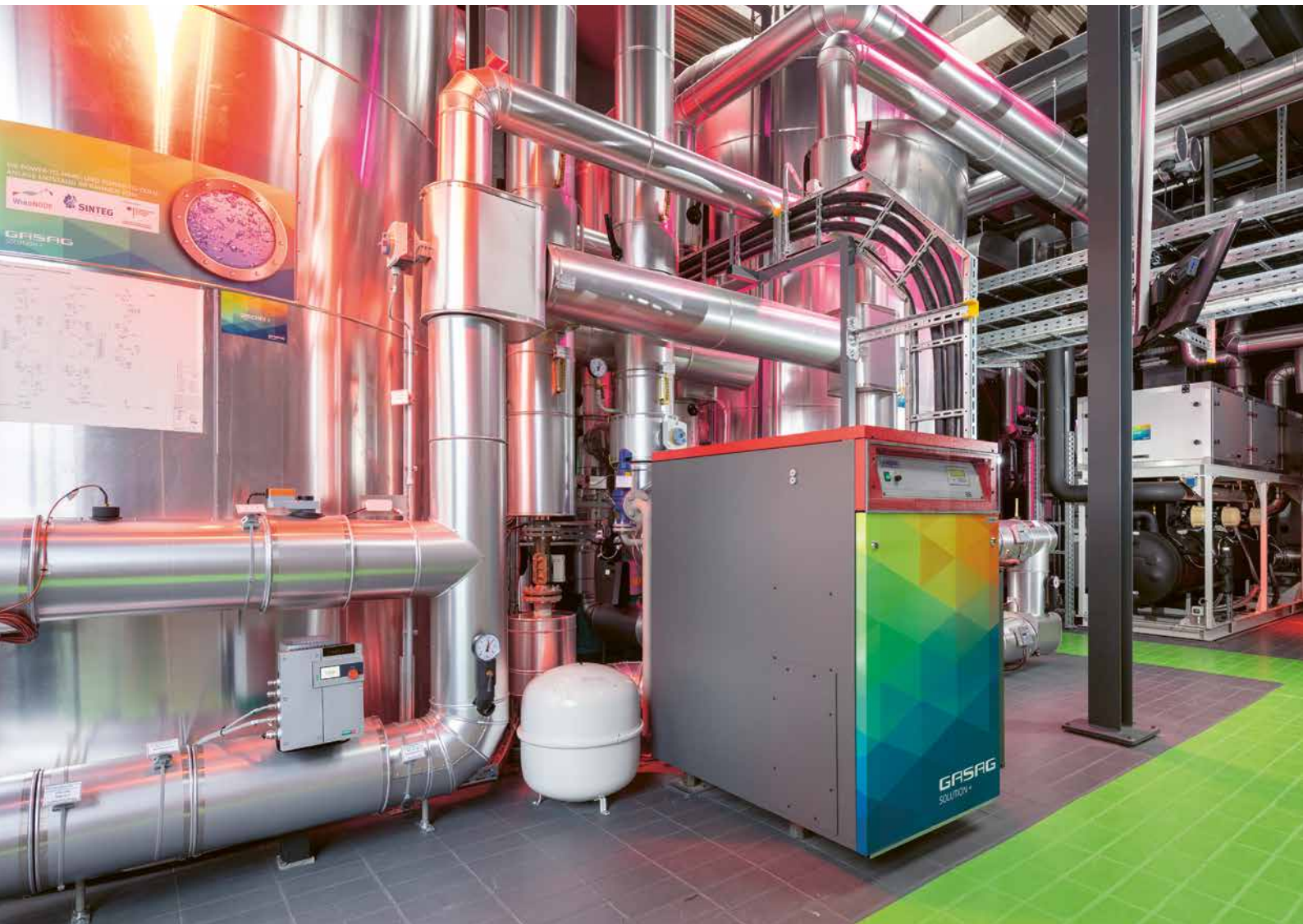
▲ A visitor site for the energy transition – Germany's first PtH/PtC plant is located in the EUREF Energy Workshop by GASAG Solution Plus.
