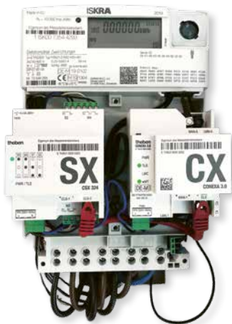
◀ Figure 3: Integrated intelligent measuring system with control box for a heat pump at the customer's premises.
