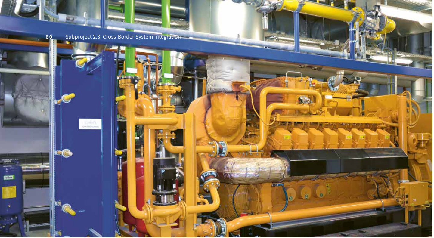
▲ Gas engine in the combined heat and power (CHP) plant in Frankfurt (Oder). The engine can generate 2,000 kW of electricity and 2,400 kW of heat.
