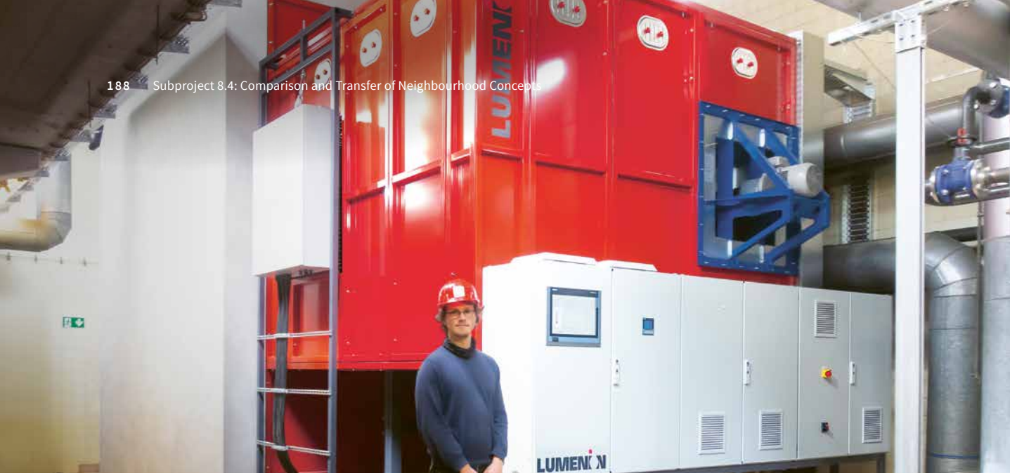
▲ The Lumenion high-temperature steel storage facility in Berlin-Reinickendorf.
