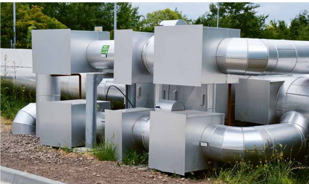
▲ Heat distribution unit in the Frankfurt (Oder) district heating grid.
