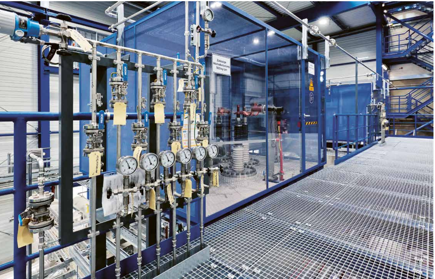
▲ Level 1 of the Power-to-District-Heating plant; view of the heads of the electrodes and a draining group.
