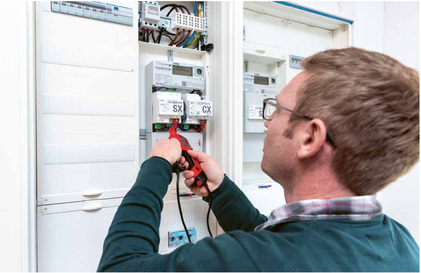
▲ Technical approval and first testing of the circuits of the first intelligent metering system with control box, which is switching the operating mode of a heat pump.
