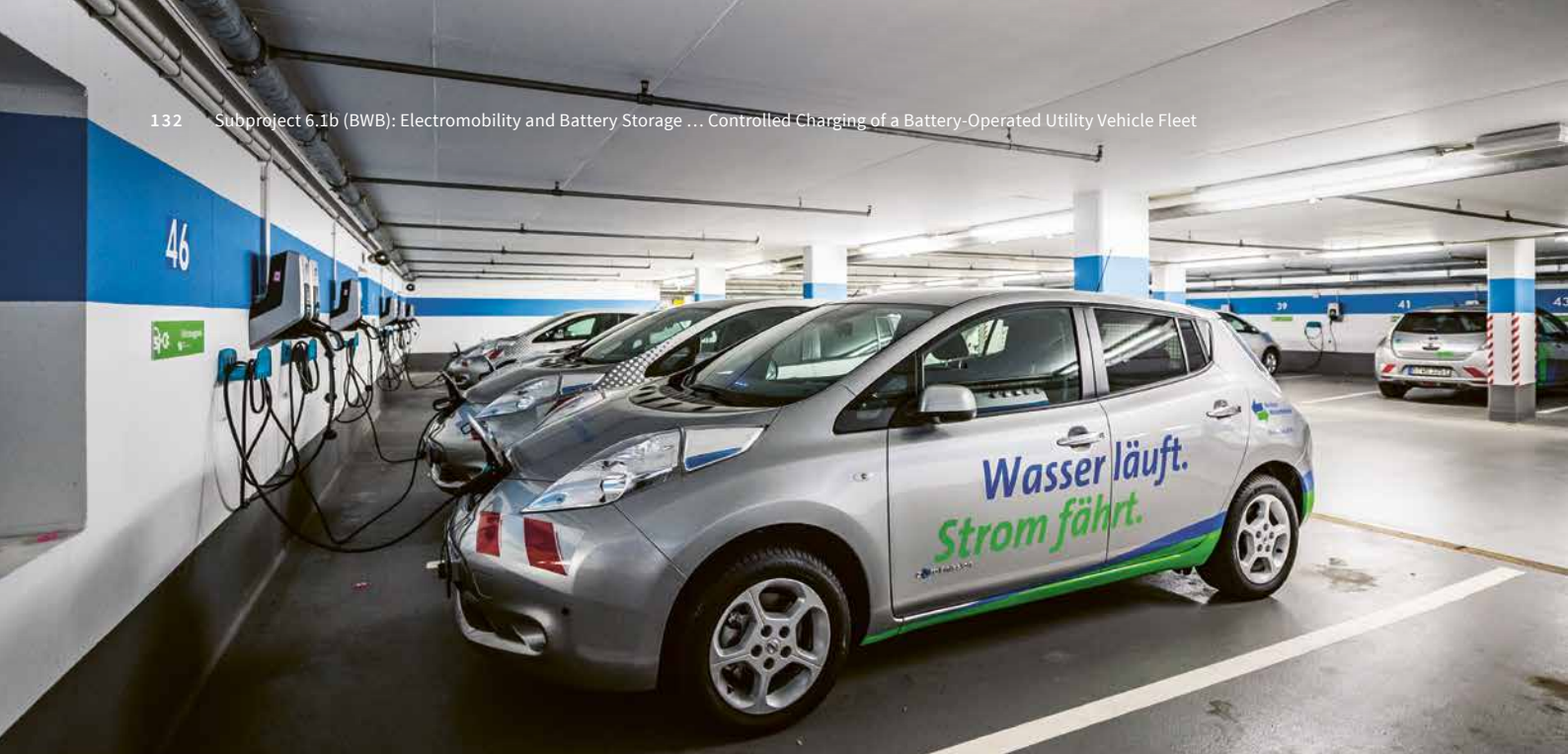
▲ Electric car in the process of charging in one of the BWB's underground car parks.
