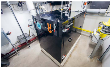
Combined heat and power unit in the boiler room
