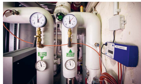
Access to local heating grid
